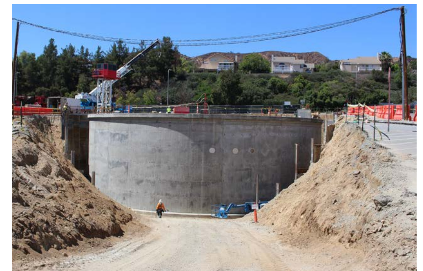
Two Million Gallon Thermal Energy Storage Tank
